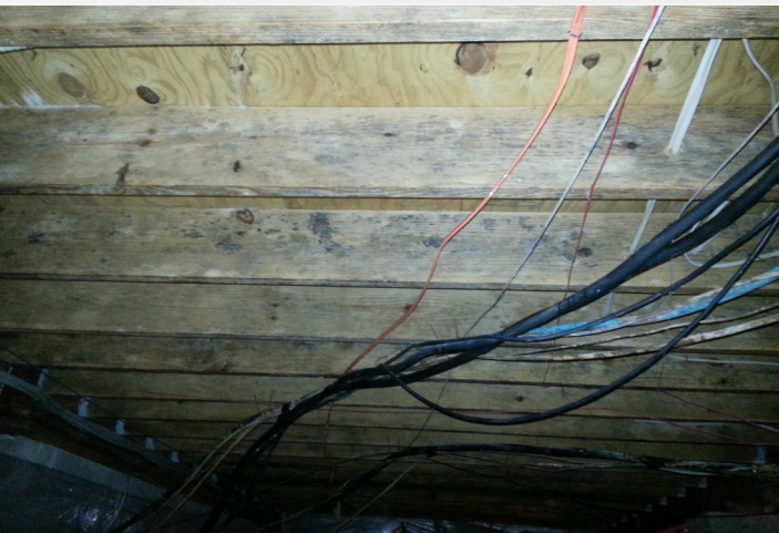
Before: Contaminated crawlspace.
